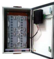
RPST with 200Ah of battery
